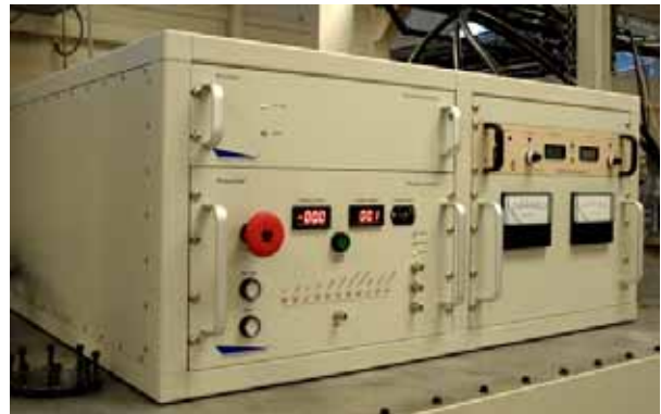
Figure 6. Modulator Controls, including fast fault detection and first fault identification.
