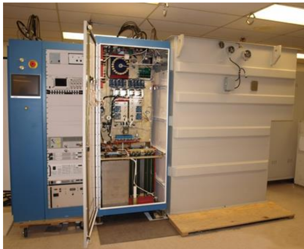
Figure 1: System designed for Oak Ridge National Laboratory Spallation Neutron Source. Design is optimized for long pulse operation with highest possible reliability and availability required for particle accelerator user facilities and test stands. High voltage cables connect to dummy load or klystrons not shown in figure.
